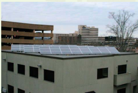
Rows of solar panels line the roof of Street Dixon Rick Architecture at 107 Kenner Avenue
